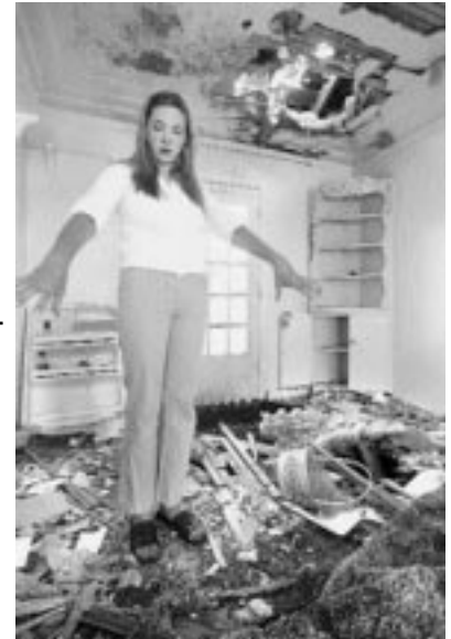
Johnna Bruner stands beside holes that an exploding water heater left in the floor and ceiling of her home.
